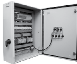
Electronic control cabinet
